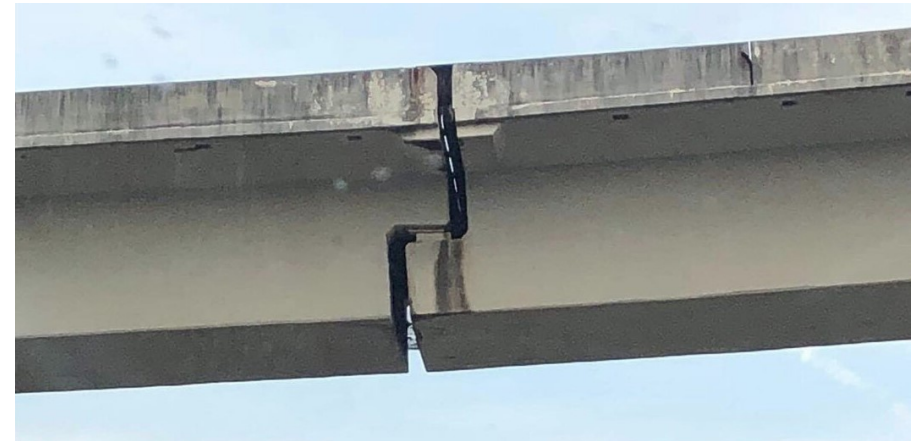
Expansion Joint failure
