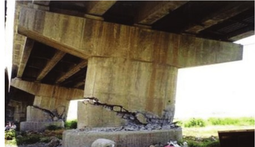
Shear failure of of substructure
